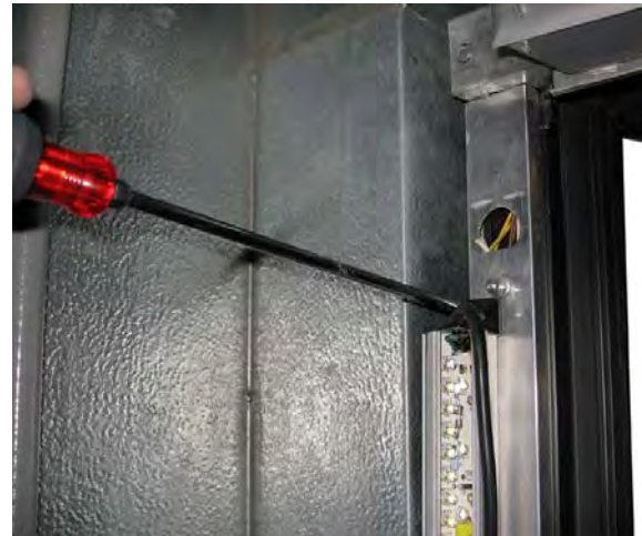
Step 4: Prepare backing tape, pre-drill, mount and screw the fixture onto the aluminum raceway.
