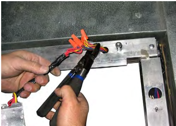
Step 3: Remove the pre-existing lighting system ballast and cut out the exposed lighting system harness.
